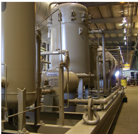
Multi-duty, multi-pass rich TEG heater for gas dehydration skid.
