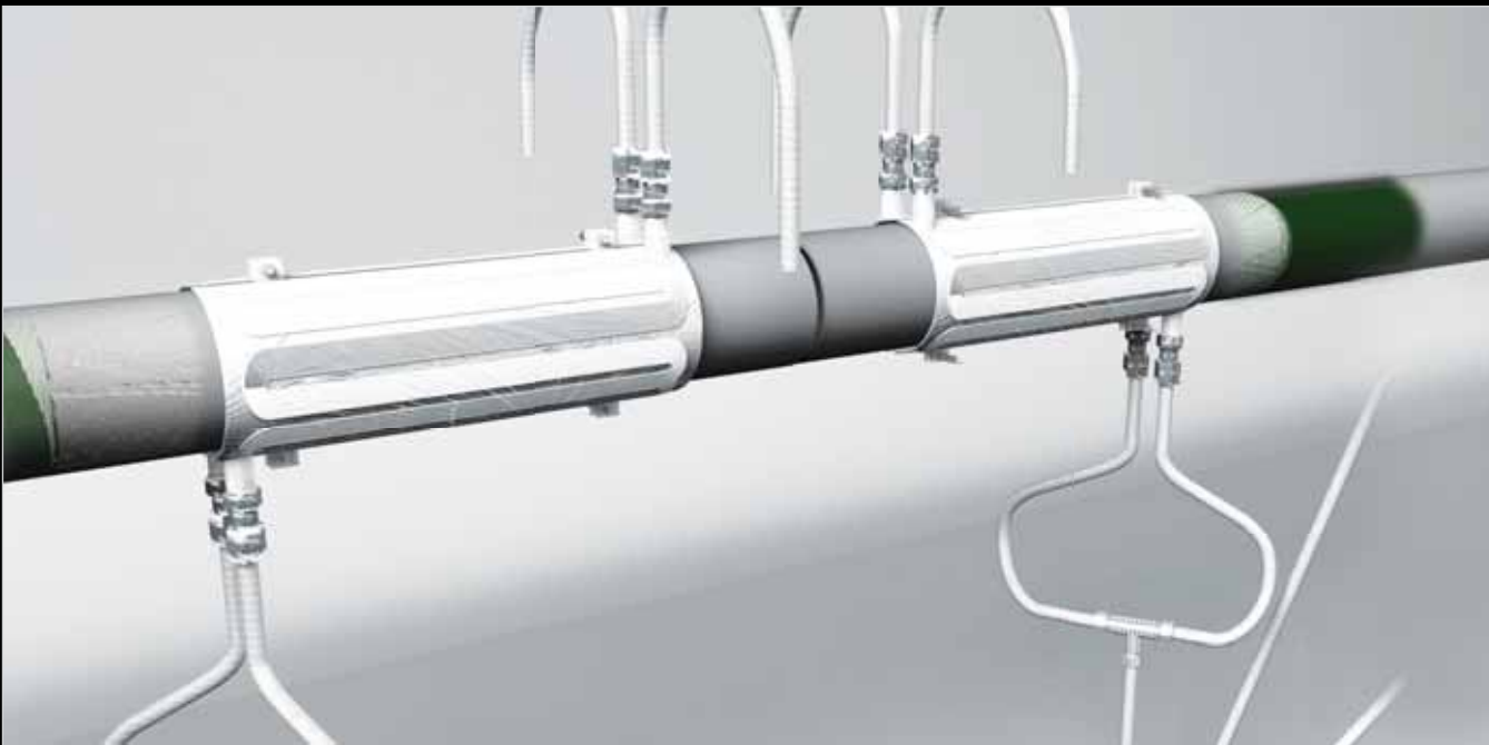
Using clamp-on PLATECOIL with cryogenic gas to freeze two plugs in a pipeline around a repair site
